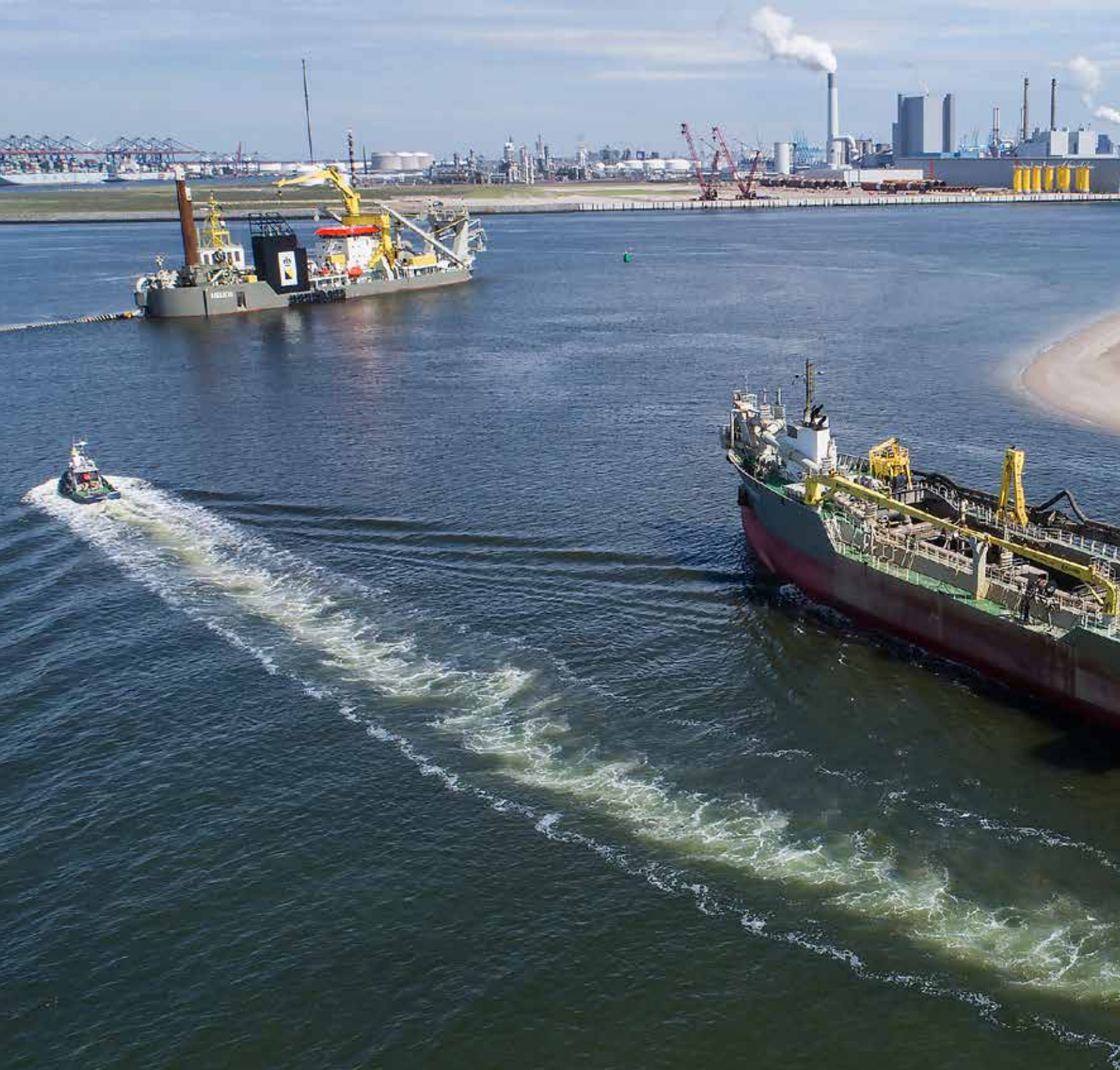
The mega cutter Helios and trailing suction hopper dredger Strandway dredging in the Port of Rotterdam.
